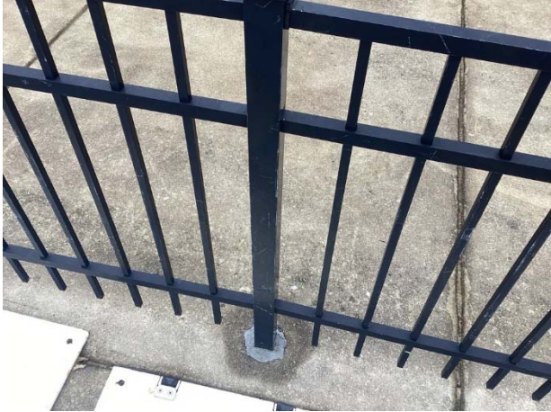
Fence finish deterioration
