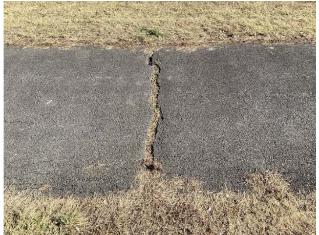
Walking path cracks
