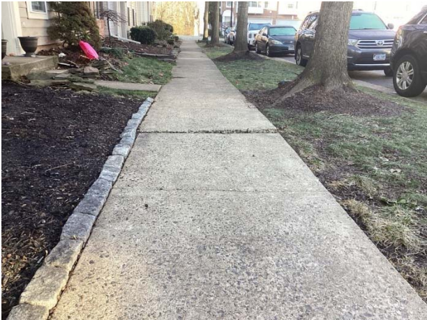
Sidewalk trip hazard
