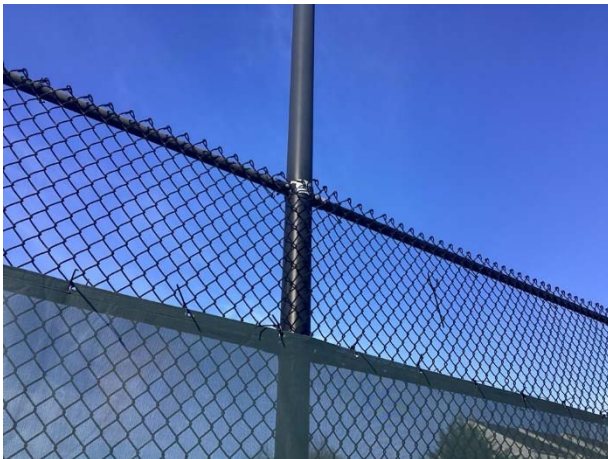
Fence finish deterioration
