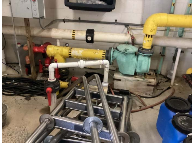
Pool mechanical equipment
