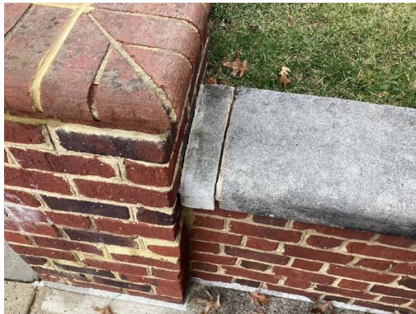
Perimeter wall mortar crack
