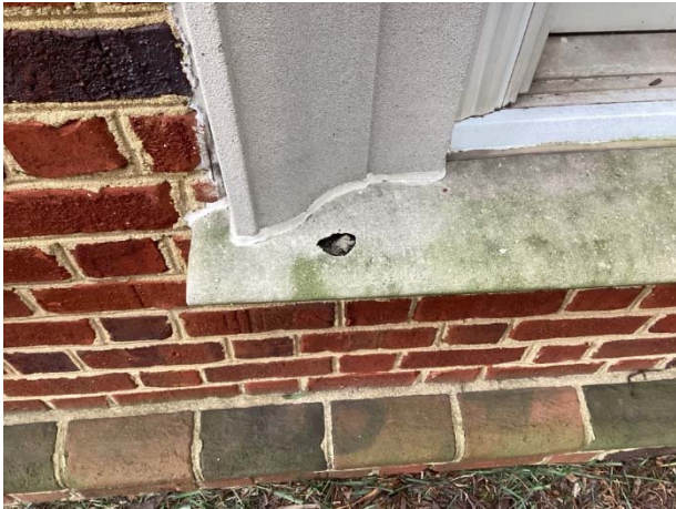
Concrete sill deterioration
