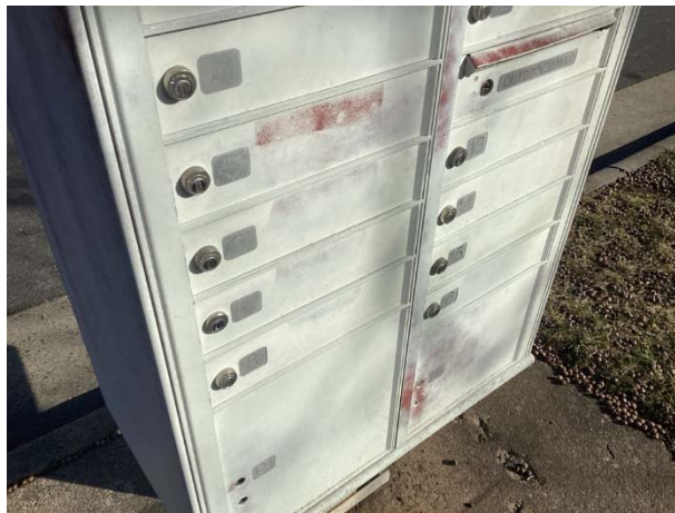
Mailbox station finish deterioration
