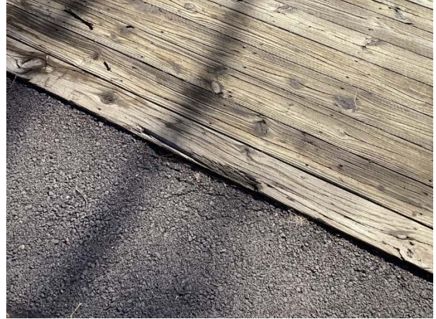
Deck board deterioration
