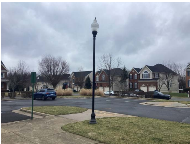
Light pole and fixture overview
