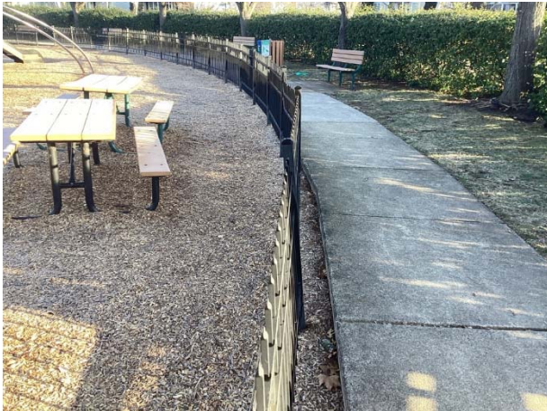
Fence leaning section
