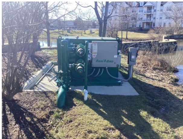
Irrigation pump system
