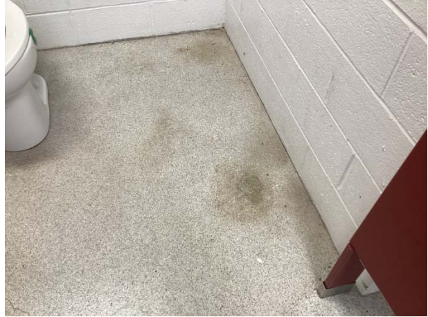
Floor coating deterioration
