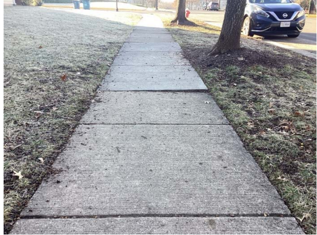
Sidewalk trip hazard
