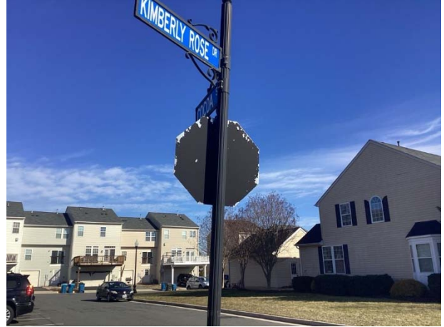
Sign finish deterioration
