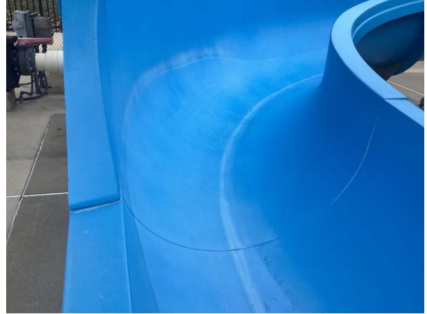
Coating finish deterioration
