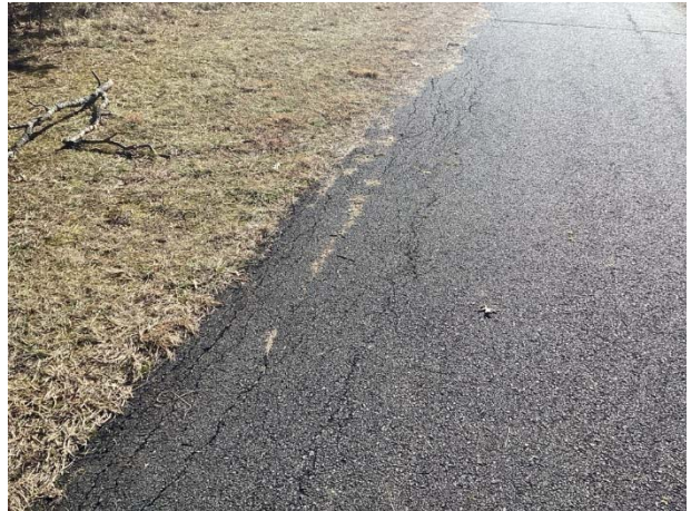
Walking path cracks
