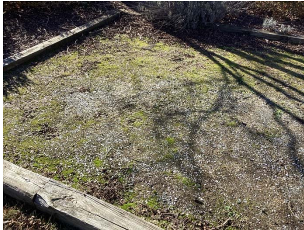
Organic growth and surface deterioration
