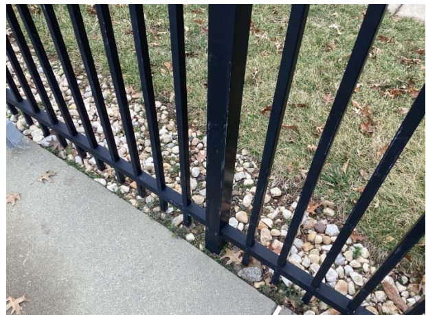
Fence finish deterioration
