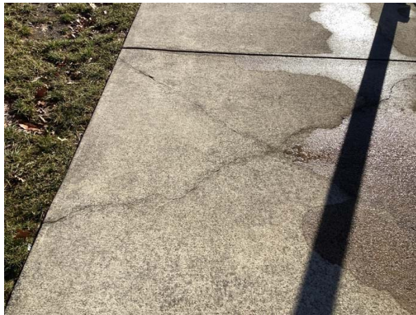
Concrete base cracks
