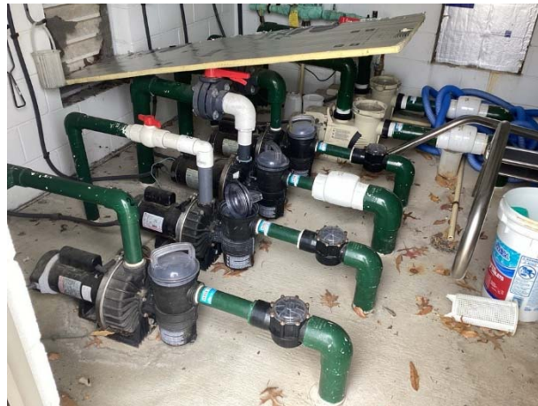
Splash pad mechanical equipment
