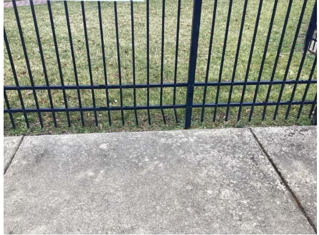
Fence picket damage
