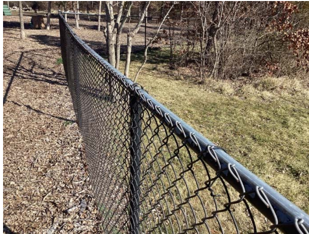
Fence finish deterioration and rust
