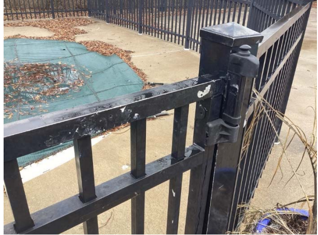
Fence finish deterioration
