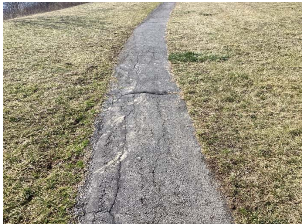
Walking path cracks
