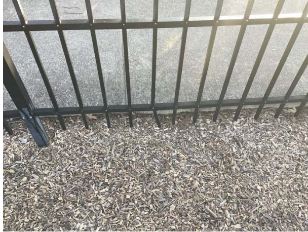
Fence picket damage
