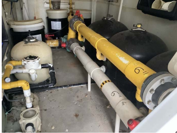
Pool mechanical equipment
