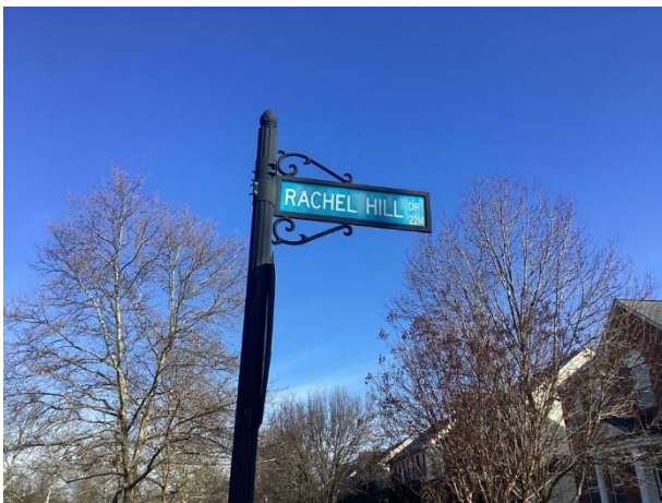
Sign finish deterioration
