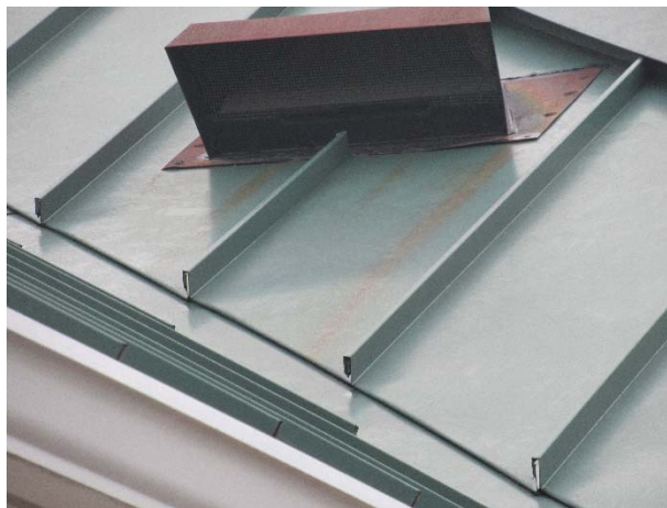
Rust stains from vent
