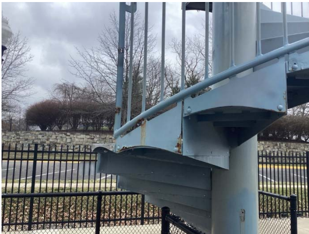
Rusted stair structure
