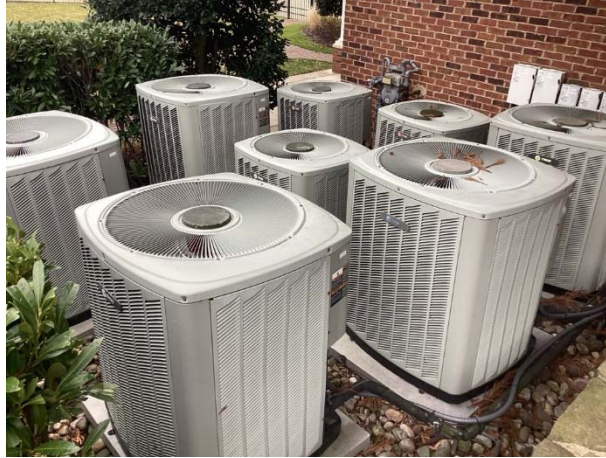
Split system condensing units
