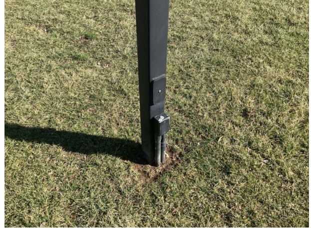
Finish deterioration and rust
