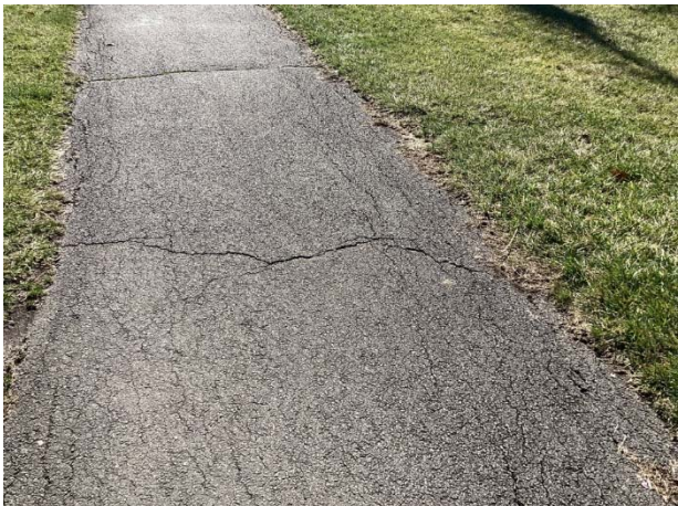
Walking path cracks
