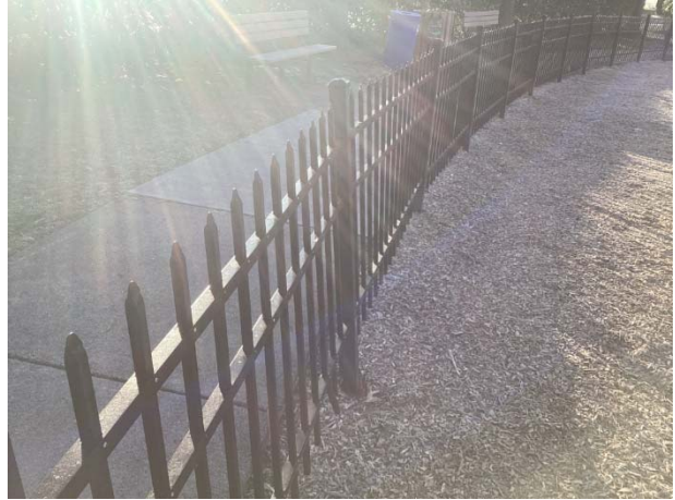
Fence leaning section
