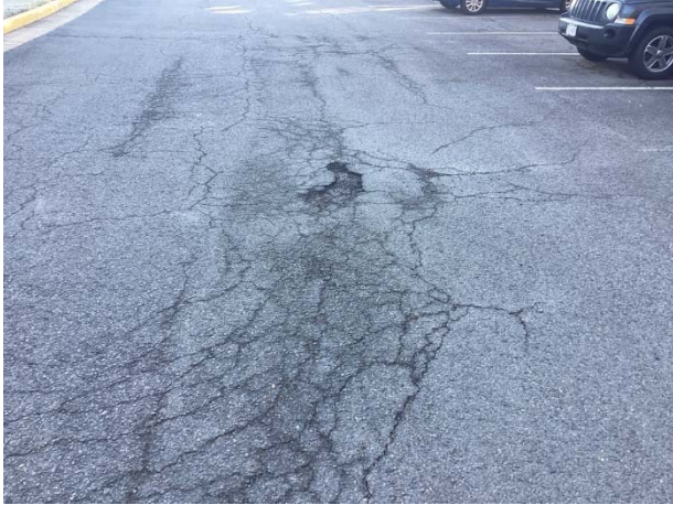
Pavement cracks and deterioration
