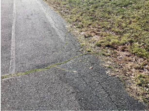
Walking path cracks
