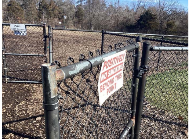
Fence finish deterioration and rust
