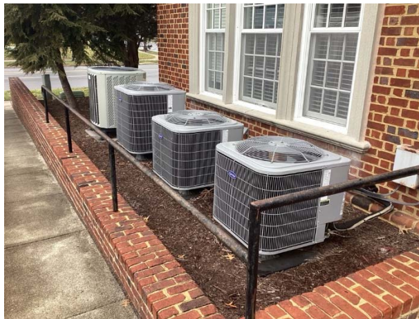
Split system condensing units
