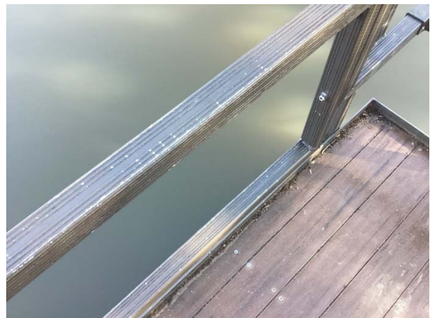
Railing finish deterioration
