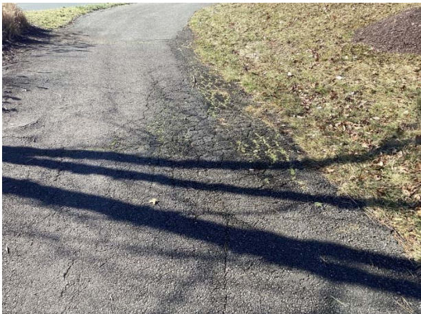
Walking path deterioration
