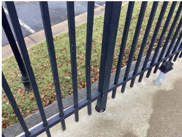
Fence picket damage
