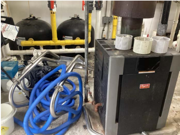
Pool mechanical equipment
