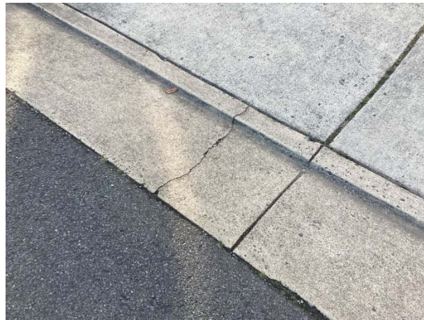
Concrete curb and gutter crack
