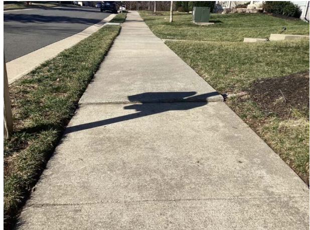
Sidewalk trip hazard
