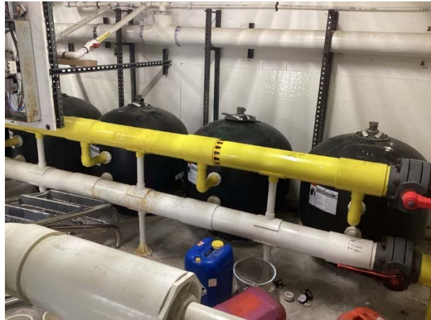
Pool mechanical equipment
