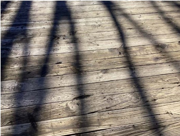
Deck board deterioration
