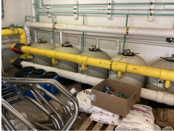
Pool mechanical equipment
