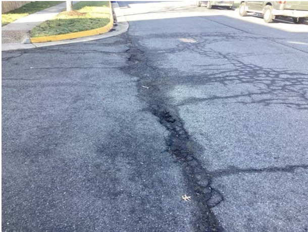
Pavement cracks and deterioration
