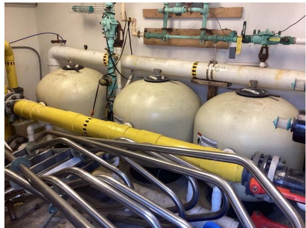
Pool mechanical equipment
