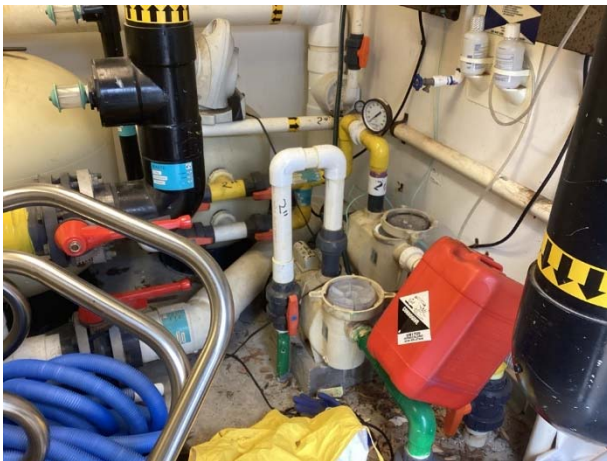
Pool mechanical equipment
