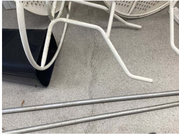
Concrete floor crack
