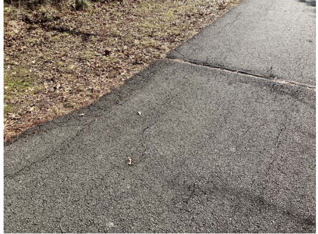
Walking path cracks
