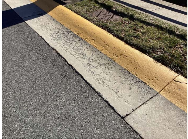
Concrete curb and gutter scaling
