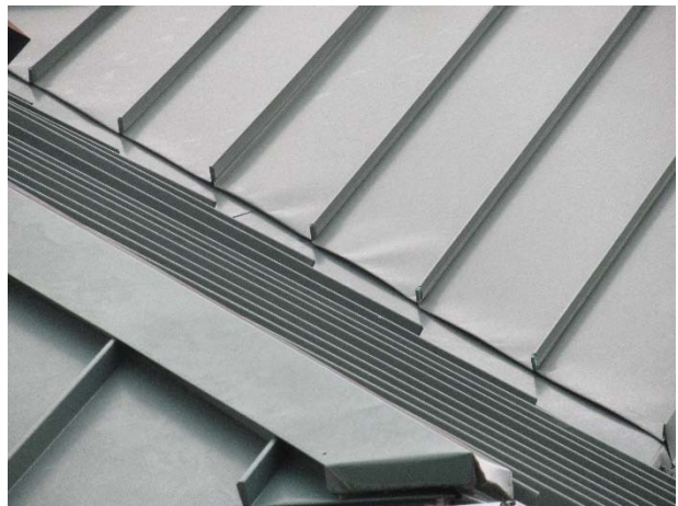
Metal roofs warp
