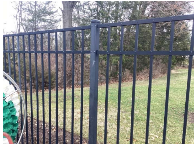
Fence finish deterioration
