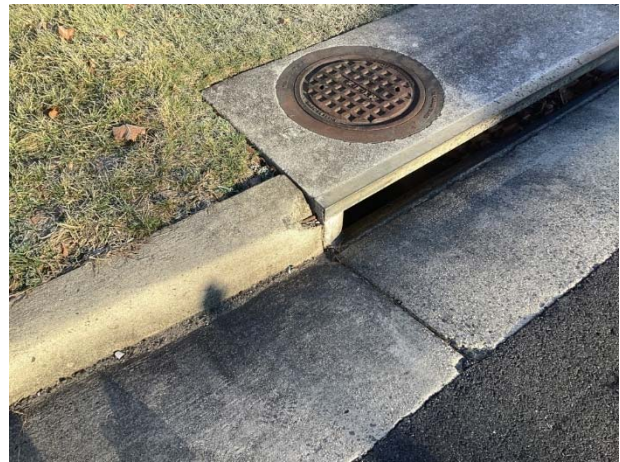
Concrete curb spall
