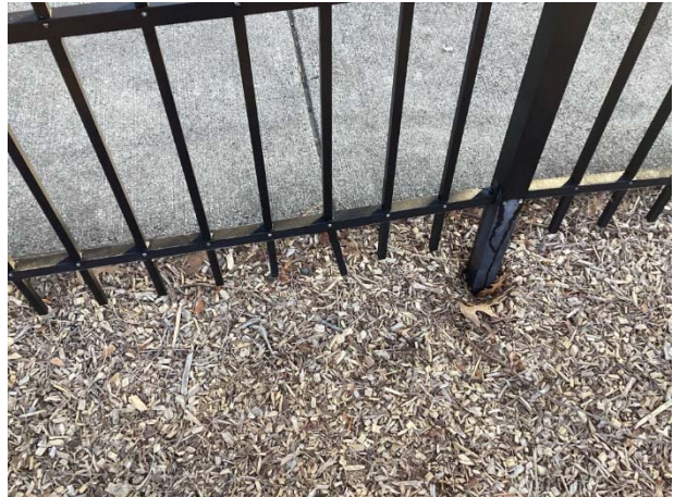
Fence picket damage
