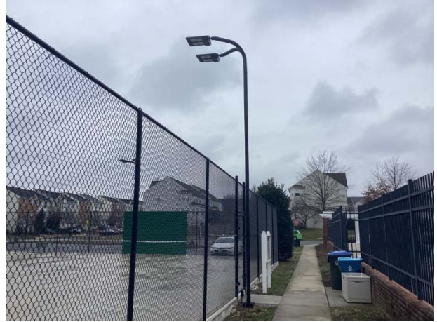
Light pole and fixtures
