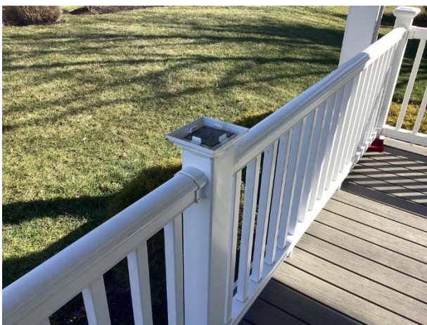
Missing railing cap
