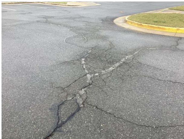
Pavement cracks and deterioration
