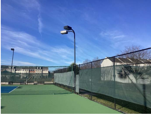
Light pole and fixtures
