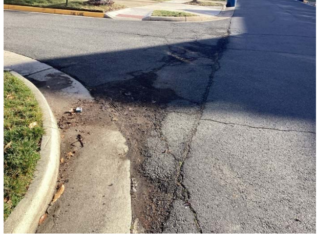
Pavement cracks and deterioration
